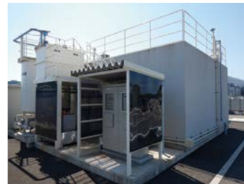
Our in-house wastewater treatment facilities
