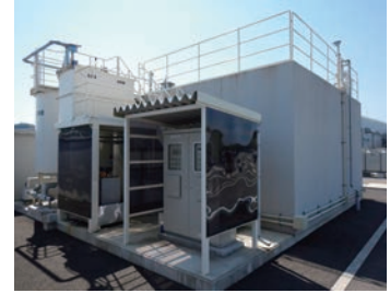
Our in-house wastewater treatment facilities
